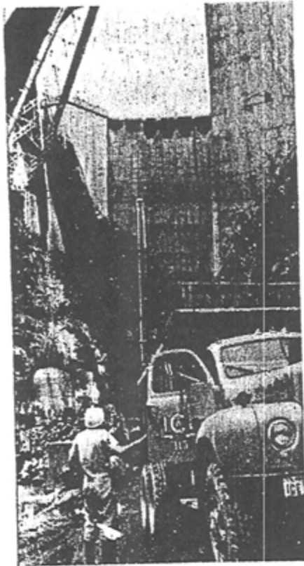
Cachi Dam, Costa Rica's largest hydroelectric project, is being built with aid of World Bank funds.
